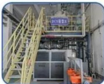
Zone of rectification
